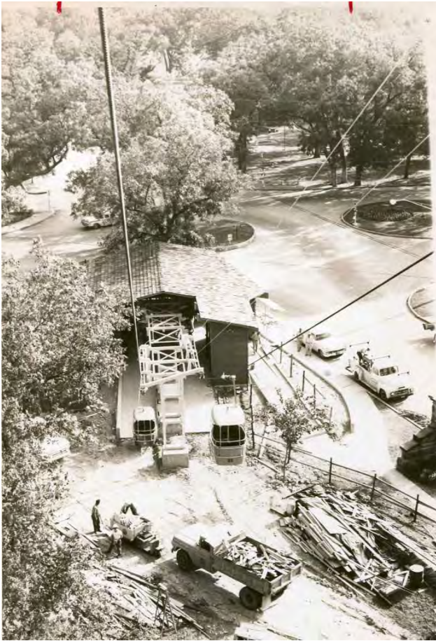
FIGURE 12–2. This image shows overhead portions of the HemisFair skyride in place, while construction continued on the infrastructure at the ground level. Source: Brackenridge Park Conservancy.
