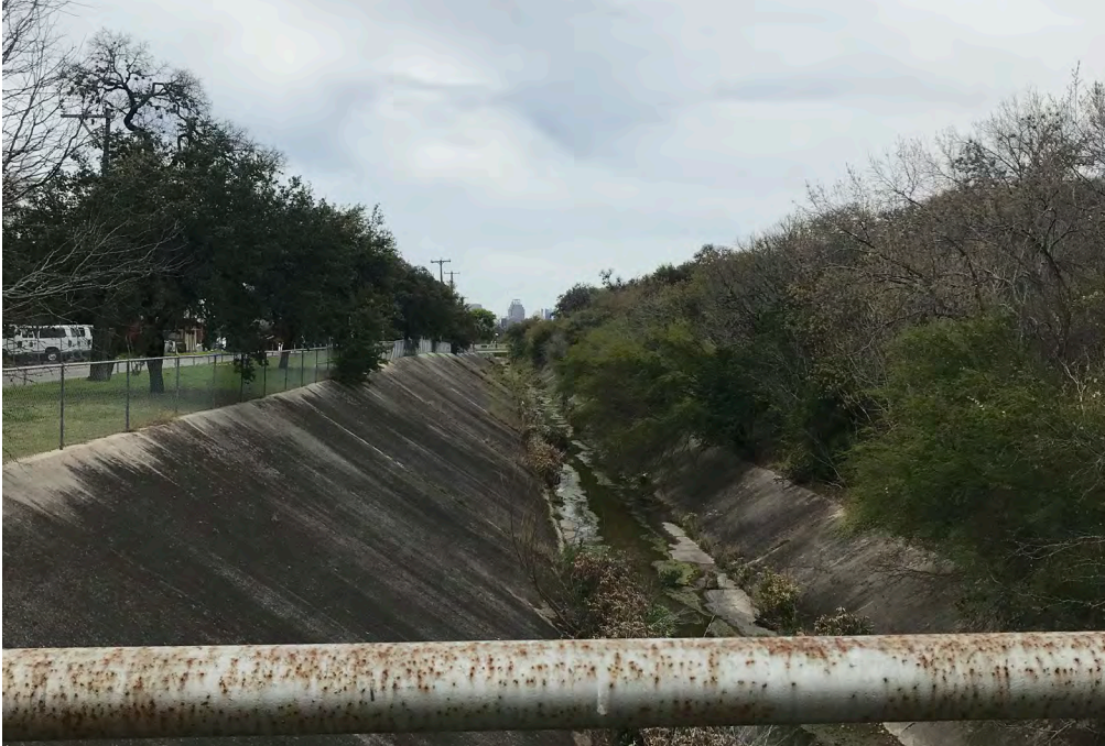
FIGURE 13–52. View of Catalpa-Pershing drainage ditch located on the west side of Avenue B. Source: Reed Hilderbrand
